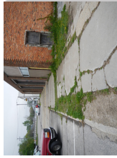
Poor Walking Surface along Railroad Street
