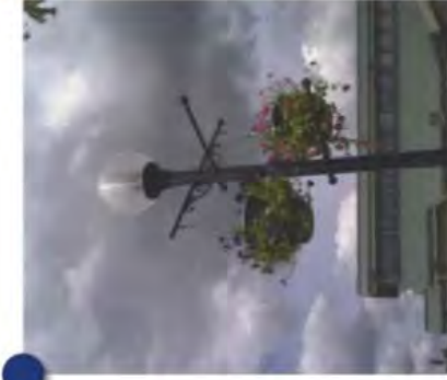
Fixture.....Metal Halide Lamp Wattage.....150 watt Number of Globes.....1
