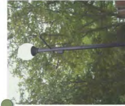
Fixture.....Metal Halide Lamp Wattage.....100 watt Number of Globes.....1
