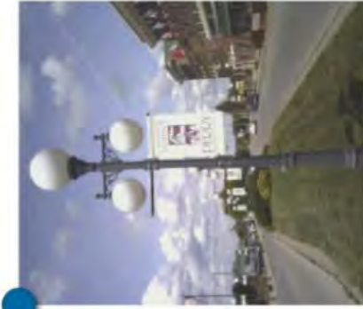
Fixture.....Compact Fluorescent Lamp Wattage.....23 watt Number of Globes.....3
