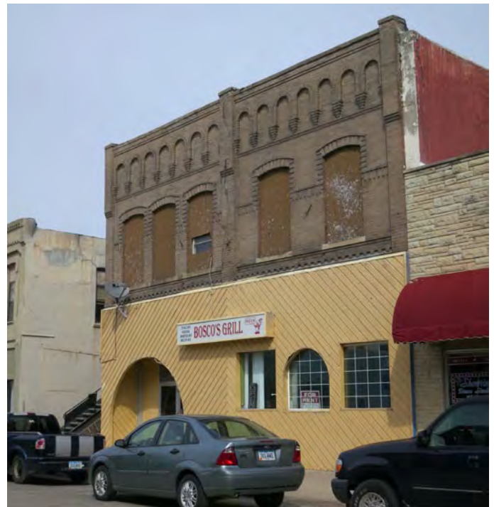
Downtown vacancy and maintenance issues
